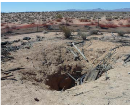
Photo of open pit, prior to clean-up activities.
