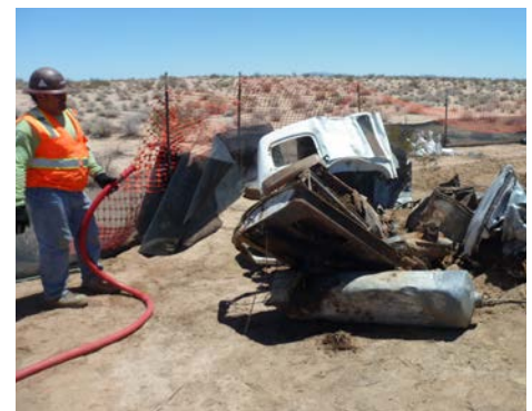
Workers use water to control dust as large pieces of cars and household debris are removed.
