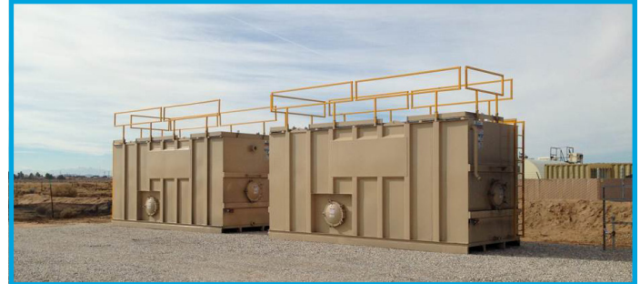
Two 10,500 gallon tanks serve as the bioreactor pilot test site.
